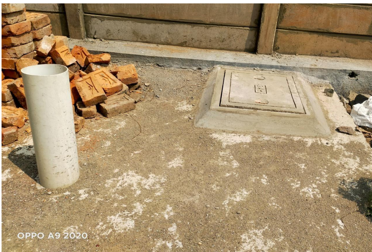
Rain water Harvesting Recharge Tube
